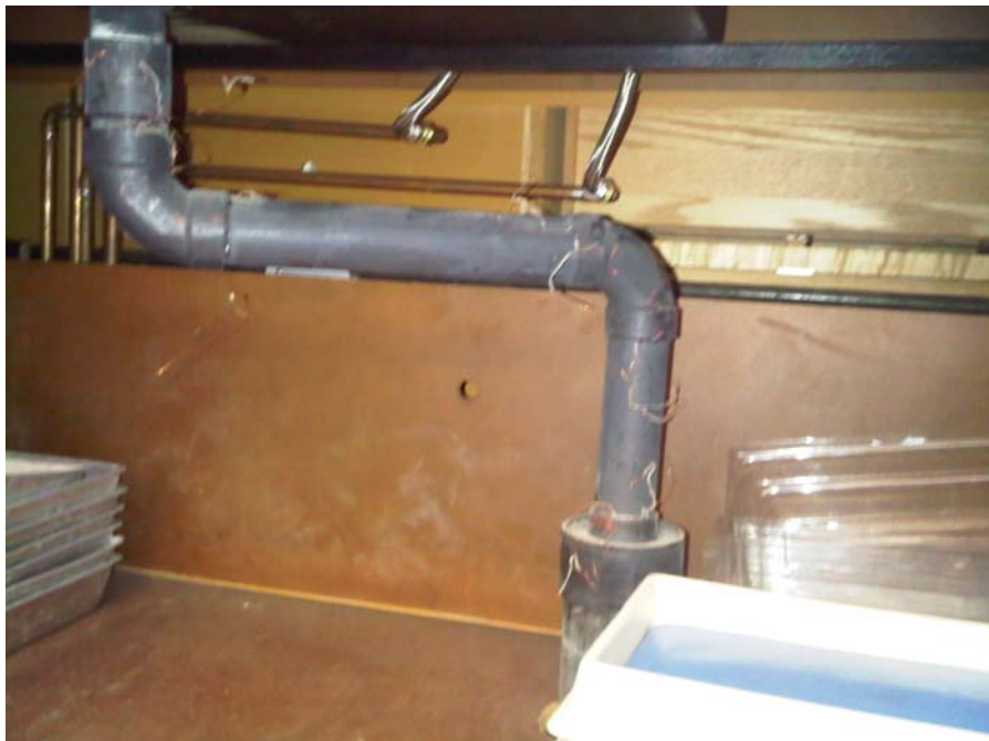
Sink trap with no "p trap". Remove piping down to floor of cabinet
